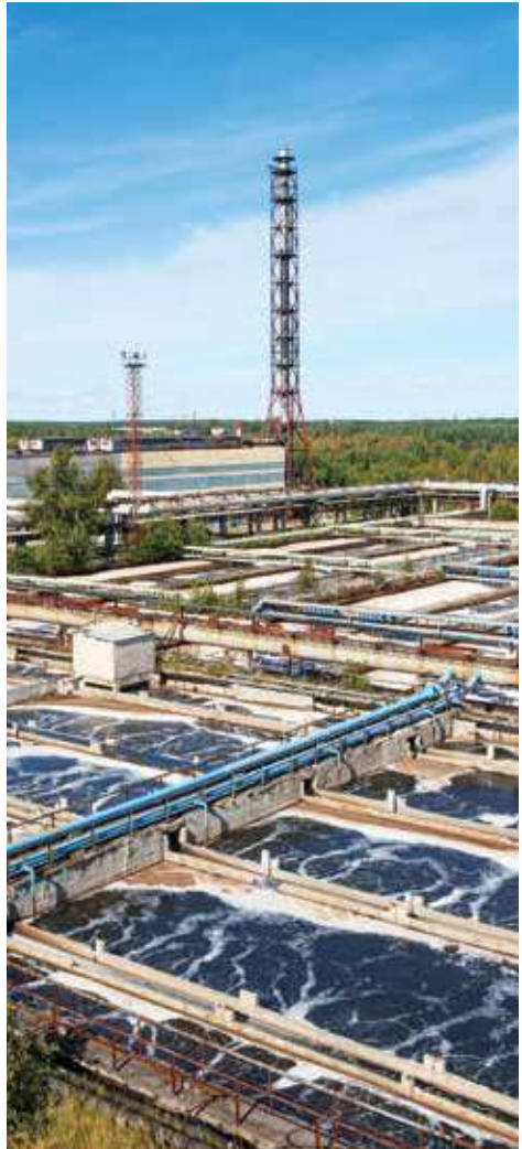
Water treatment facility
