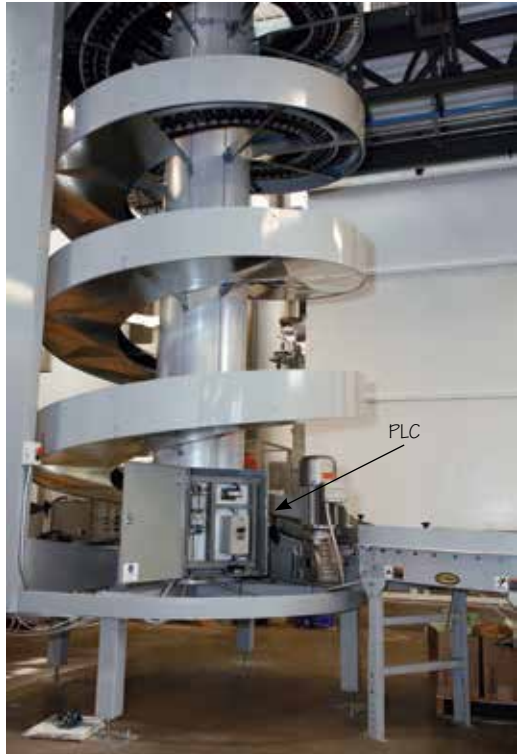
This PLC controls motors and sensors in an automated distribution facility, including this spiral conveyor system.
